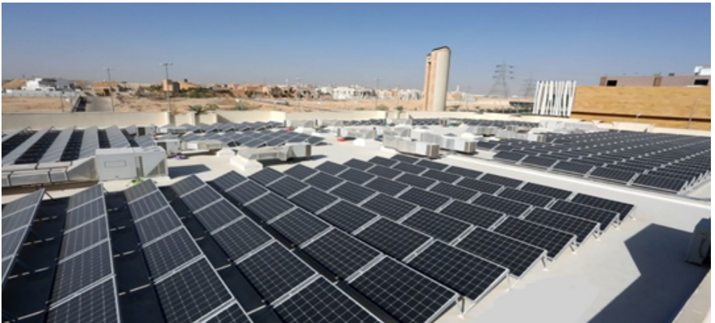
Figure 5. The installed and commissioned 124 kW solar PV system on the mosque's rooftop.
